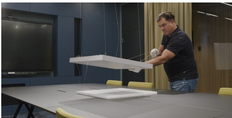
The Sennheiser ceiling microphone was supplied, installed and set up by Supravisio AG
